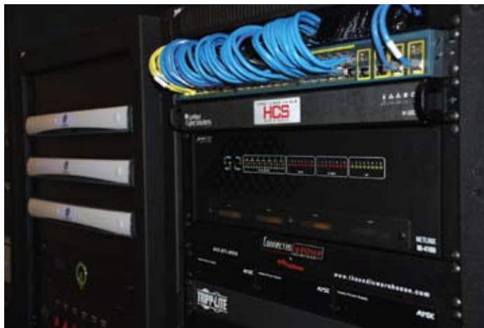
The Home Cyber Shield H-100, a single-rack-space server, deployed at the Kiawah Island home
